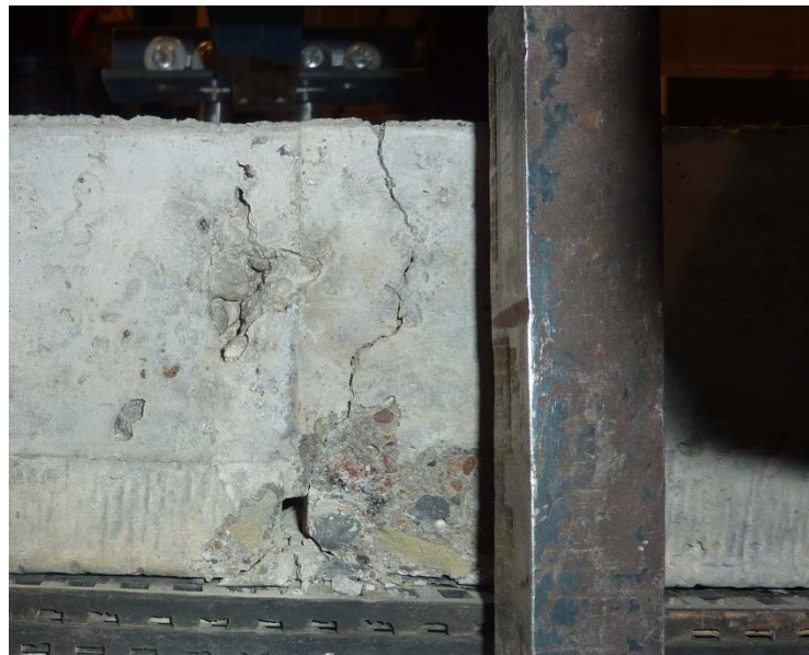
Figure 5.50. Crack profile near the loading location for the PC slab, side view.
