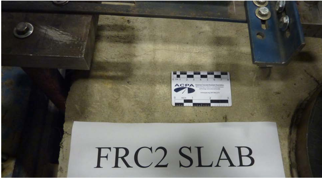
Figure 5.67. Initial crack width of FRC2 slab before the starting of the joint performance test, top view.
